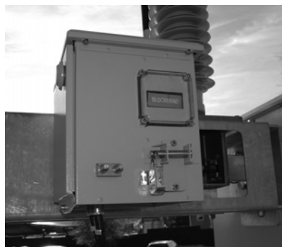
Figure A1.5. The disconnecting circuit breaker is locked in open position. The sign indicates blocked [32]
